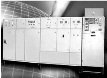
Test Panel Up to 11KV
